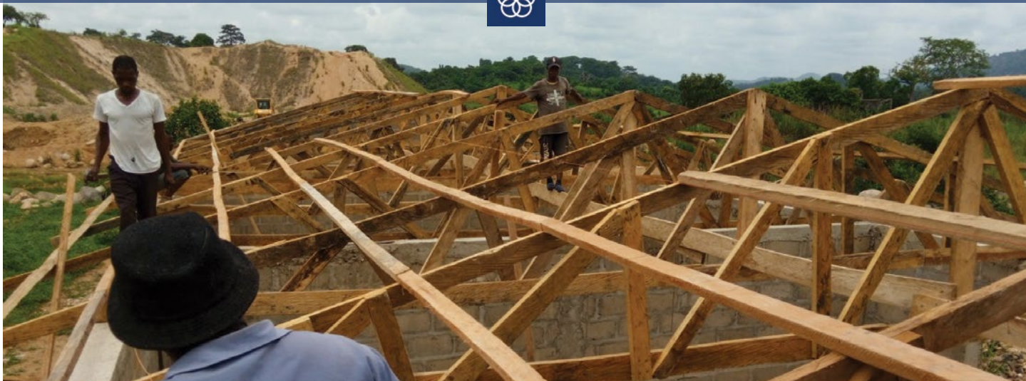
Accountable Development Works/Sierra Leone Action Mission Committee: Koidu Academy School Construction progress in Sierra Leone.
